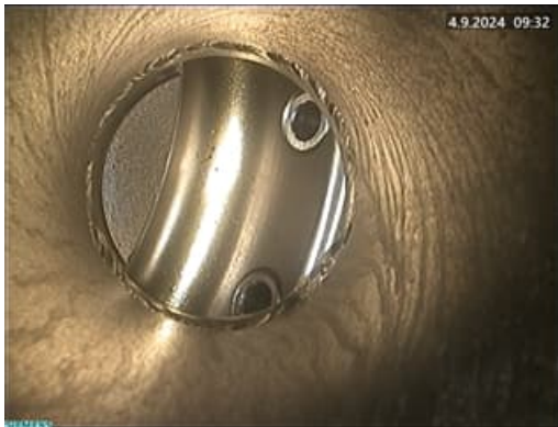
Burner #14 Premix gas passage
