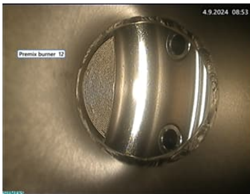
Burner #12 Premix gas passage
