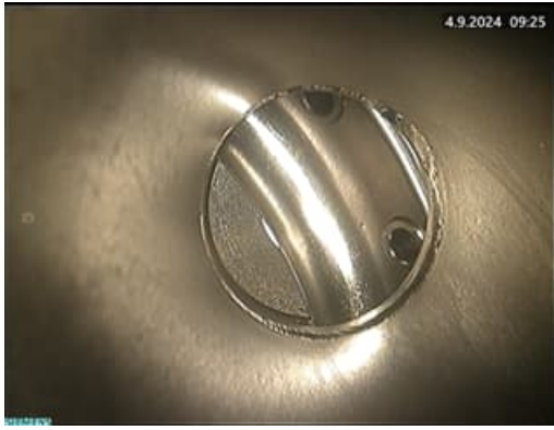
Burner #10 Premix gas passage
