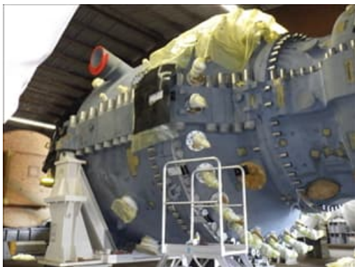
LHS turbine side
